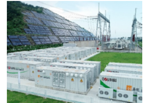
Haifeng AGC Energy Storage and Frequency Conversion Project
